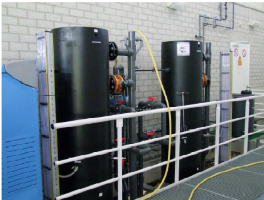
Figure 7-2 GAC columns used in pilot plant at Dunea
