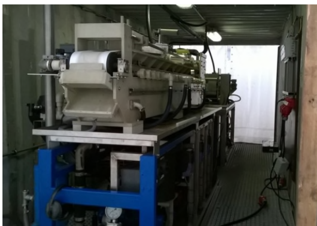
FIGURE 2-3 ONE OF THE SEPARATION UNITS
