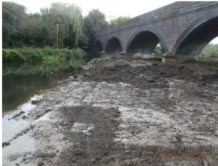
Figure 4 After increasing river flow capacity at the Great Central Way Biam Bridge.
