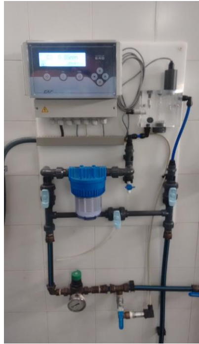
Figure 43 Chlorine analysis equipment.
