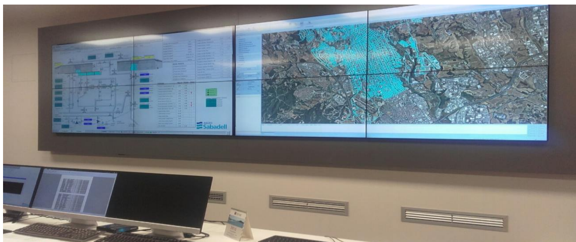
Figure 48 Control room in Sabadell.
