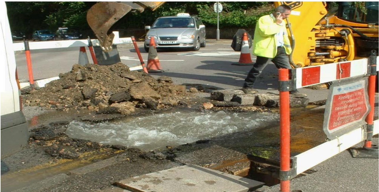
Figure 65 The detected leak within 1m of model prediction
