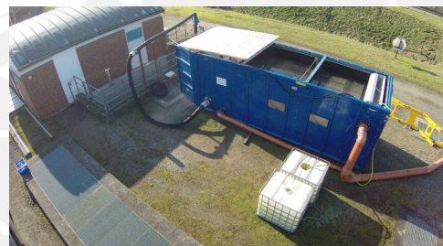
Lamella settler container solution at CSO facility
