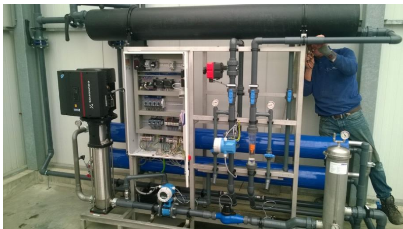
Figure 48: Installation for infiltration and recovery of the rainwater (top) and the desalination of water recovered with high salinities (via the Freshkeeper) (bottom).
