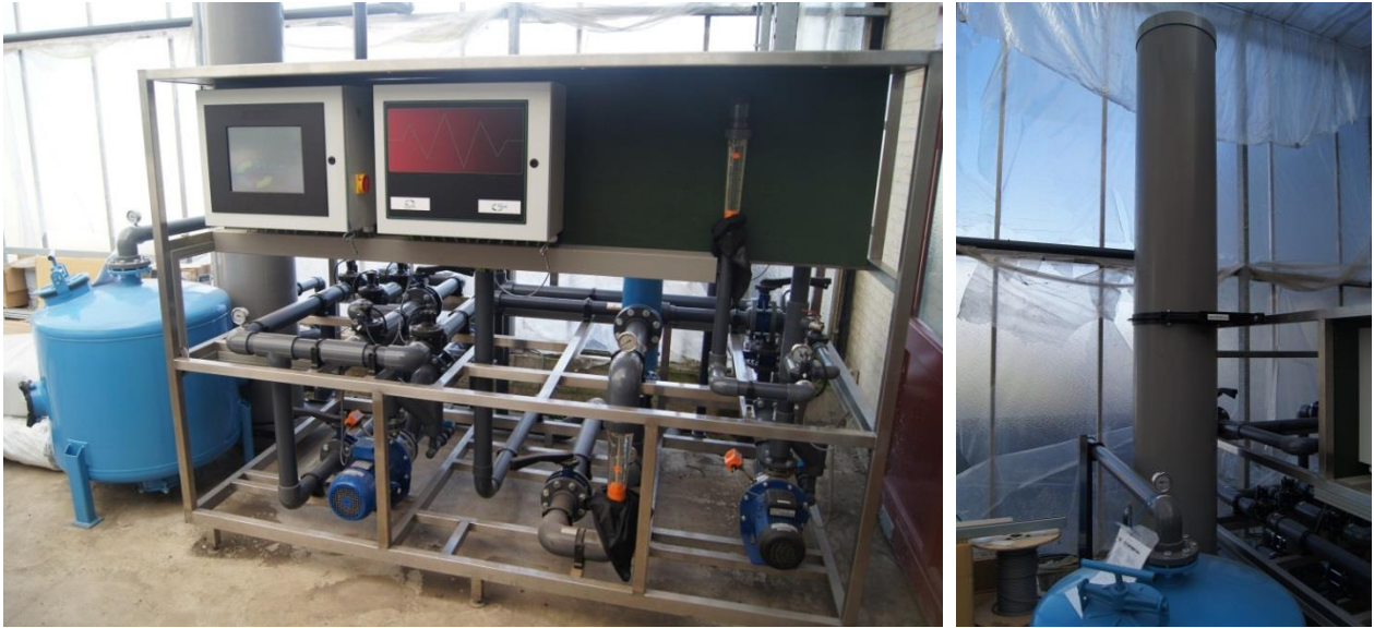
Figure 8: ASR pump and control unit, including the rapid sand filter (blue tank) and the pressure standpipe used to provide a constant pressure for infiltration (right).
