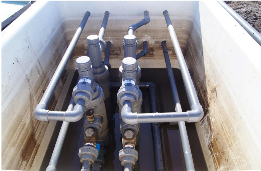
Figure 6: Multiple partially penetrating well heads at ASR-Coastal Nootdorp
