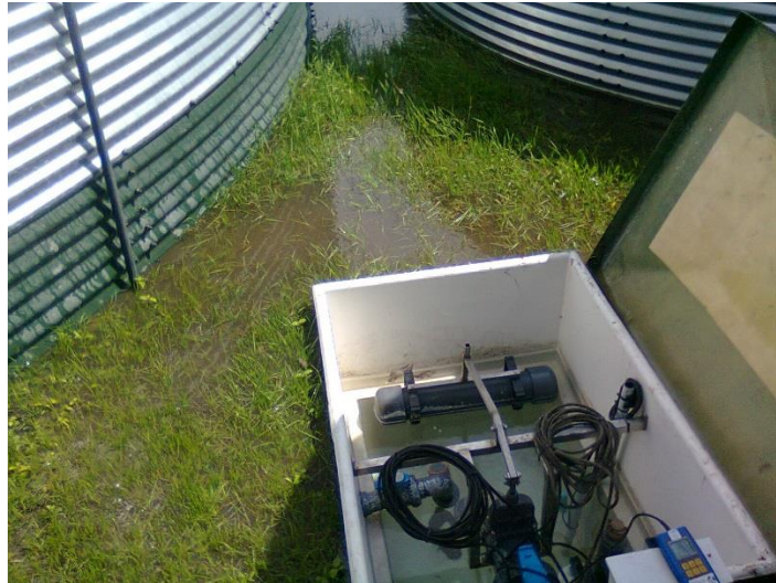
Figure 36: Rainwater in the low area around the floater box of the slow sand filter.
