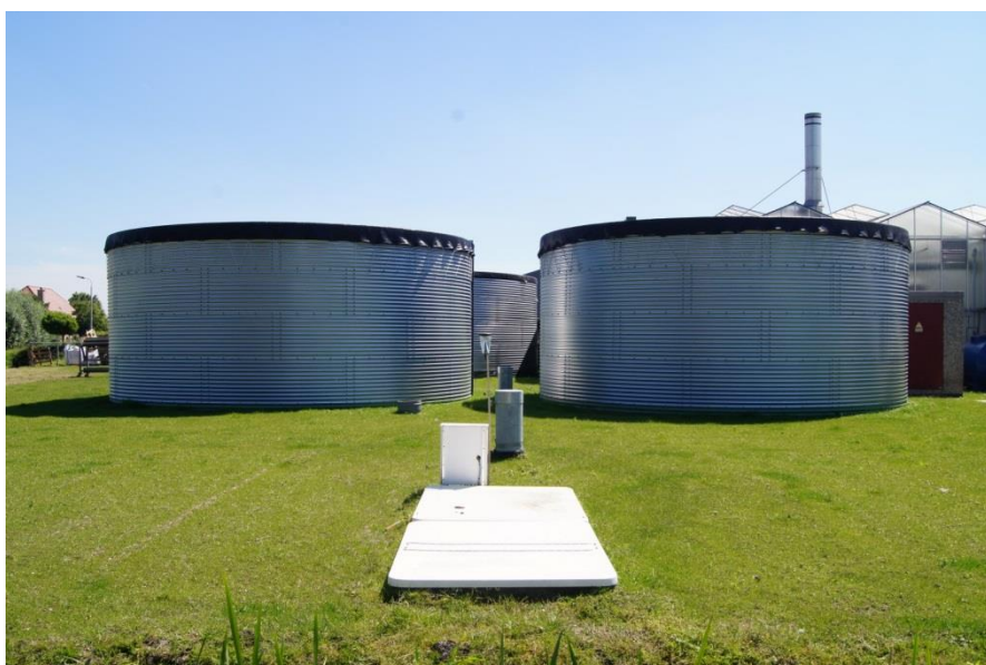
Figure 5: ASR-Coastal well field Nootdorp: infiltration well and monitoring equipment in front (white covers), and monitoring wells (steel cases) and storage tanks (one for rainwater, others for water reuse) in the background.
