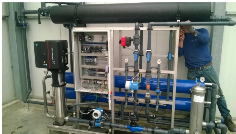
Figure 10.6: Installation for infiltration and recovery of the rainwater (top) and the desalination of water recovered with high salinities (via the Freshkeeper) (bottom).
