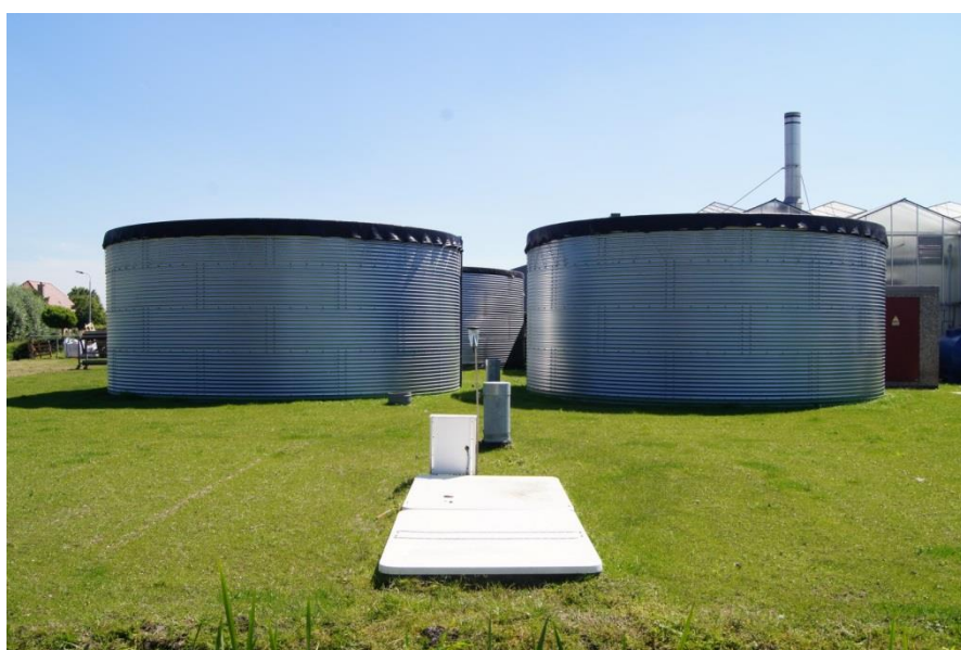
Figure 2.5: ASR-Coastal well field Nootdorp: infiltration well and monitoring equipment in front (white covers), and monitoring wells (steel cases) and storage tanks (one for rainwater, others for water reuse) in the background.
