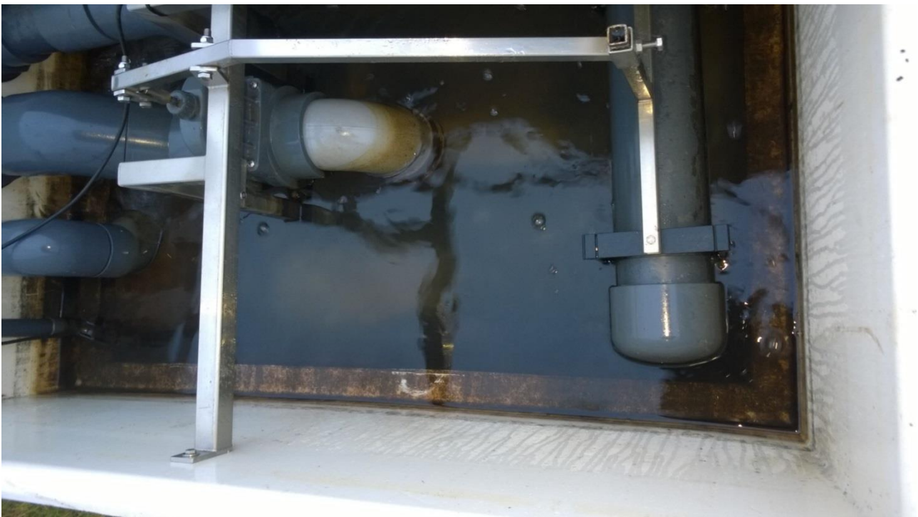
Figure 17.1: Biogrowth in the floater box at ASR-Coastal site Westland
