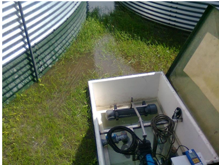
Figure 8.1: Rainwater in the low area around the floater box of the slow sand filter.
