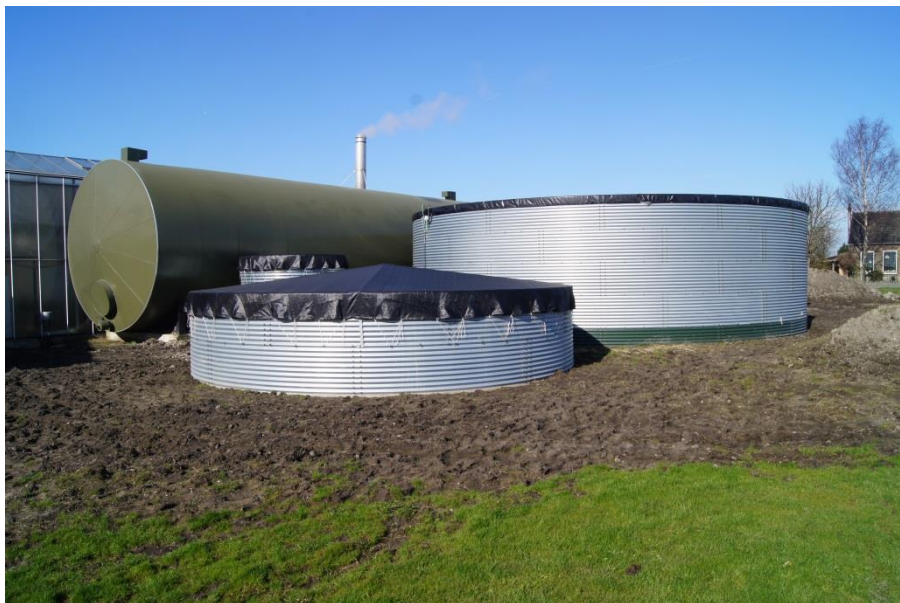
Figure 2.7: Tank of the of the slow sand filter (left) and the rainwater storage tank (right). Green tank is for heat storage, not water supply.
