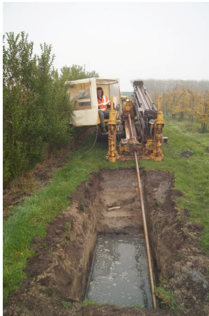
Figure 2-3 Installation of the horizontal directional drilled wells (HDDW) for the Freshmaker in Ovezande (Zuurbier et al., 2015).
