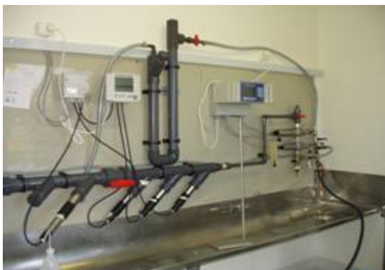
Figure 1. The measurement station in Dösebacka.
