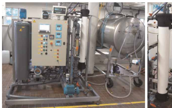
Figure 1 | The pilot-scale FO set-up and the SWFO membrane module at the KWR pilot facility in Nieuwegein.
