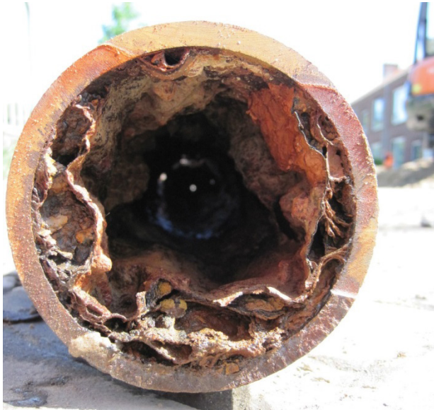
Figure 4.2 Example of corrosion in CI-pipe.
