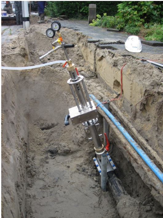
Figure 4.3 Example of a situation in which cables were causing problems with the use of the balloon valve.
