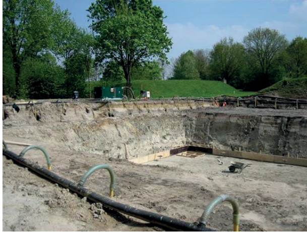
Fig. 1.3 Construction dewatering in practice: groundwater lowering at an excavation site by using a vacuum well-point system.
