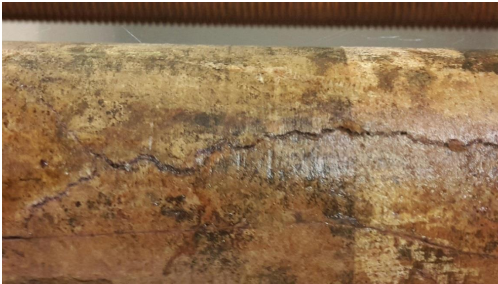
Figure 3.1.4.2: The cracked pipe.
