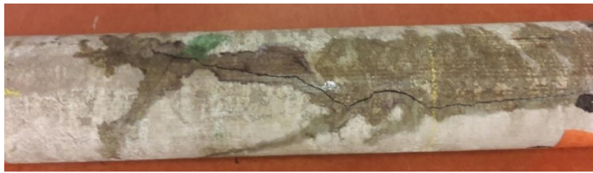
Figure 3.1.9.2: The cracked pipe.
