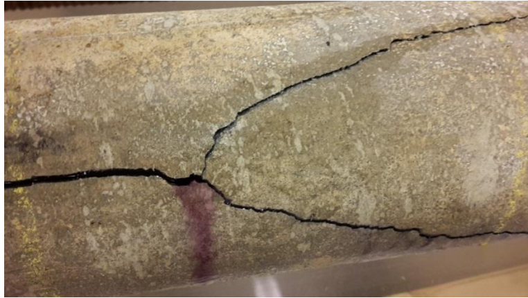
Figure 3.1.1.2: The cracked pipe.
