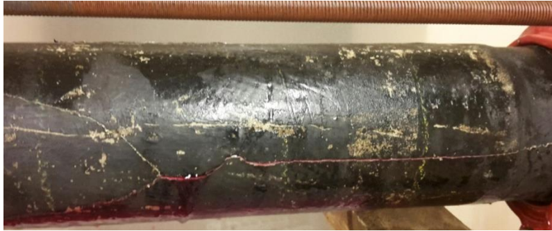
Figure 3.1.15.2: The cracked pipe.
