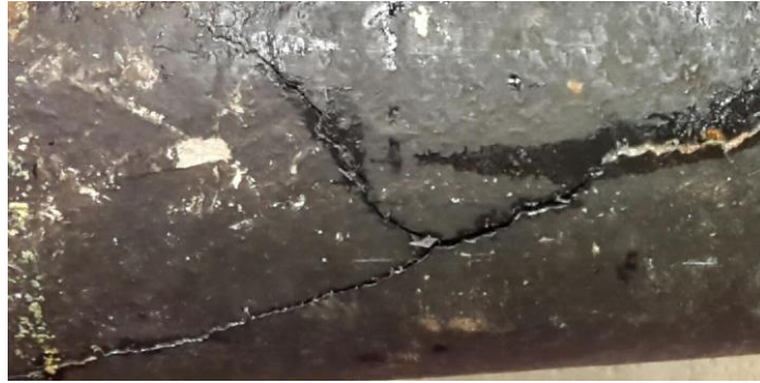
Figure 3.1.2.2: The cracked pipe.
