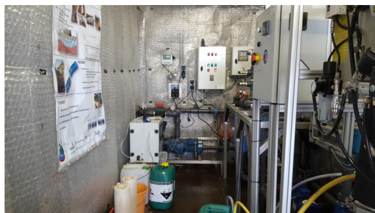
Figure 21 Test setup of the BACTcontrol at Ovezande
