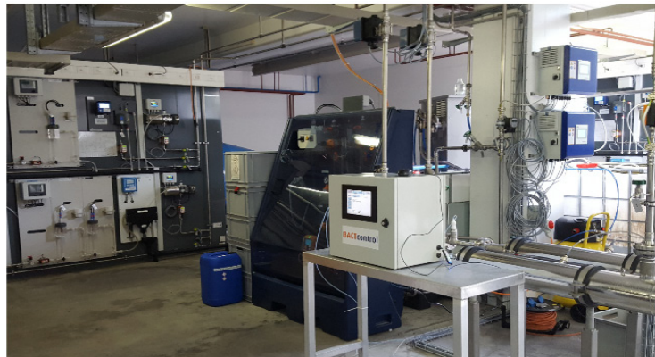
Figure 13 View of the BACTcontrol device installed at the Lange Erlen pilot plant.
