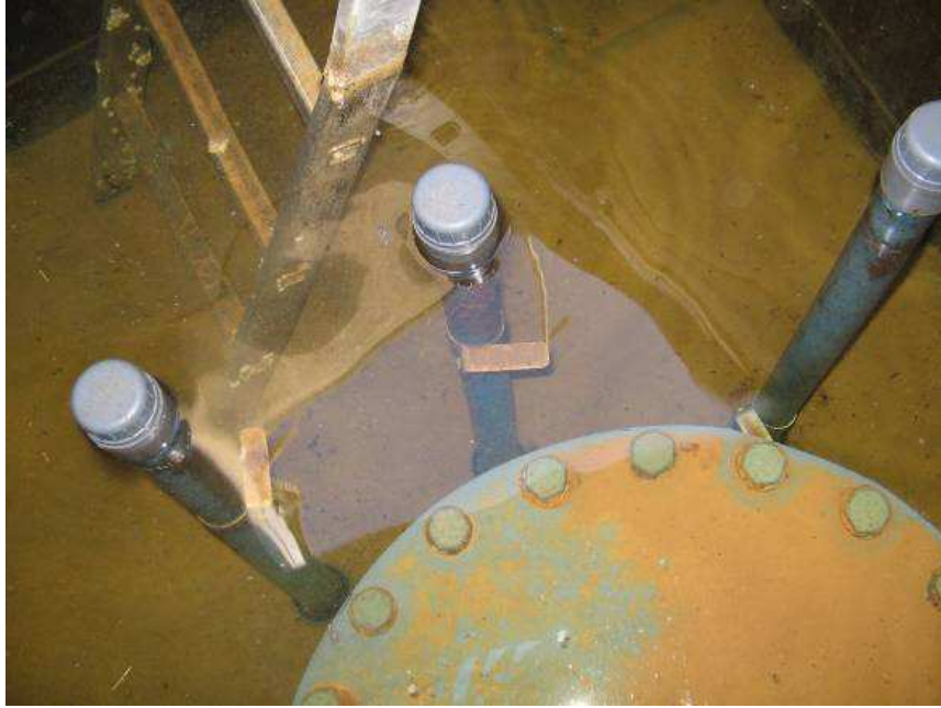
Figure 3.6 Flooded well head. The water level is above the well top, but just below the top of the observation wells (piezometers). Protective caps will prevent flood water from entering the observation wells and short-circuiting of this water to the well screen. Photo courtesy of water supply company Brabant Water, the Netherlands.
