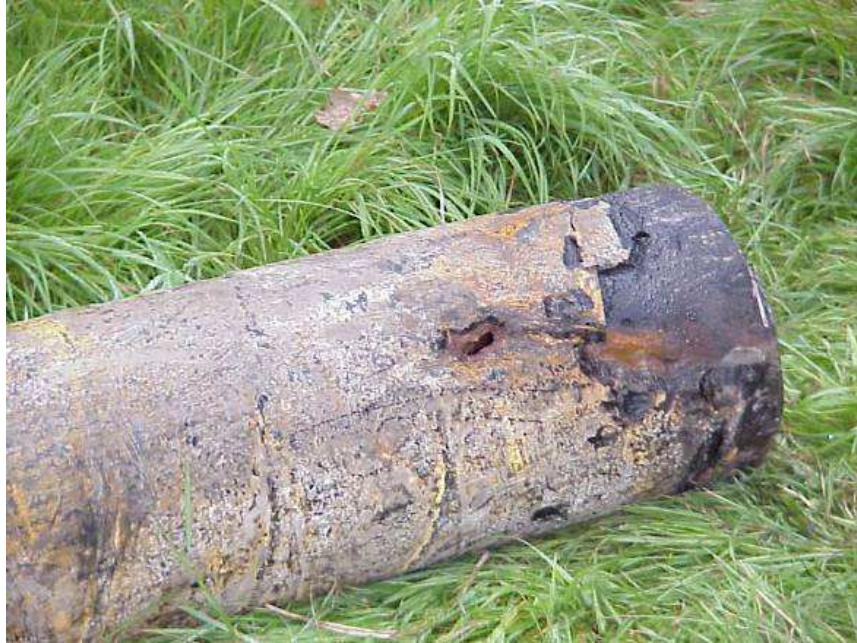
Figure 3.8. A heavily corroded stainless steel casing. The holes provide a short-circuit route for infiltrating flood water. Photo courtesy of water supply company Oasen, the Netherlands.
