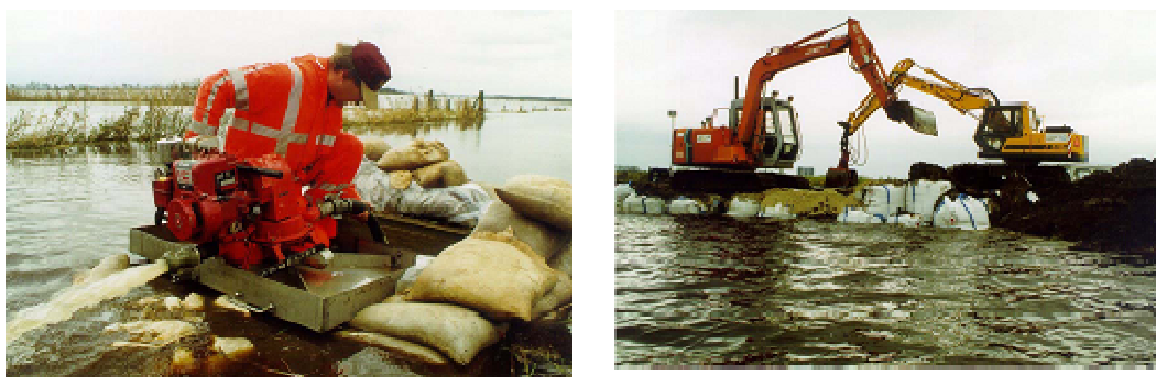
Figure 4.3 Protection by sand bags of a production well (left) and the pumping station (right) in Onnen, the Netherlands. Photos courtesy of water company Groningen, the Netherlands.
