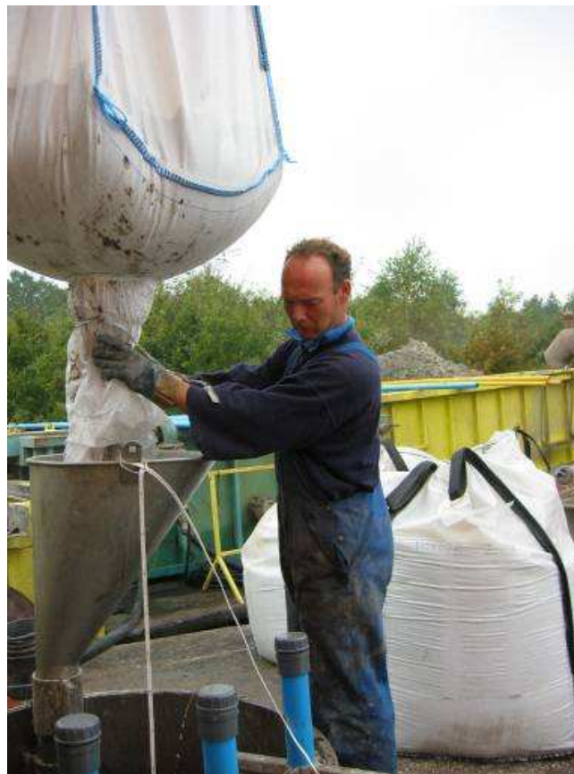
Figure 3.7 A bentonite clay seal is installed during construction of a new water abstraction well. Photo courtesy of water supply company Brabant Water, the Netherlands.
