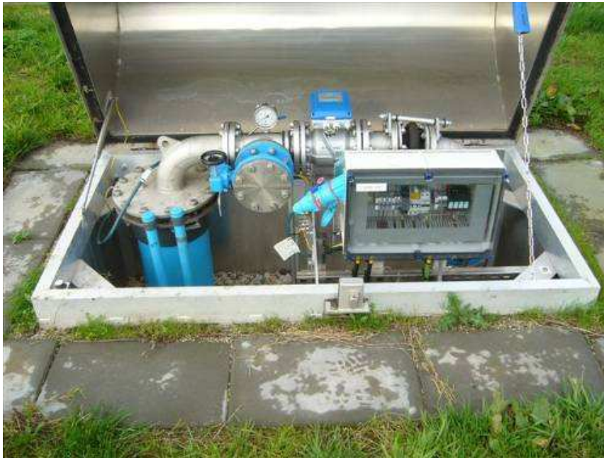
Figure 3.5 Well head interior, including the well cover, observation well(s), and electrical system. This well was installed on an artificial mound and thus protected from flooding. Photo courtesy of water supply company Groningen, the Netherlands.
