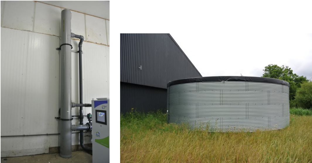
Figure 3: Standpipe to provide infiltration pressure (left) and buffer (right)
