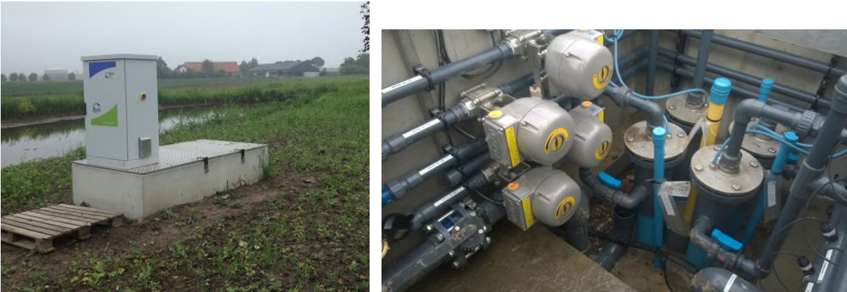
Figure 7: The first ASR-well (PP1) in the well field in Dinteloord (left) and its well completion including control valves in the well house (right)
