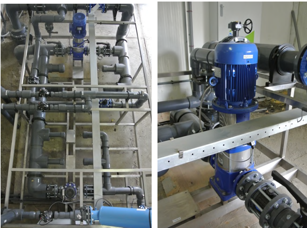
Figure 4: Topview of the Dinteloord ASR-facility and close-up of the booster pump for supply to the distribution loop.
