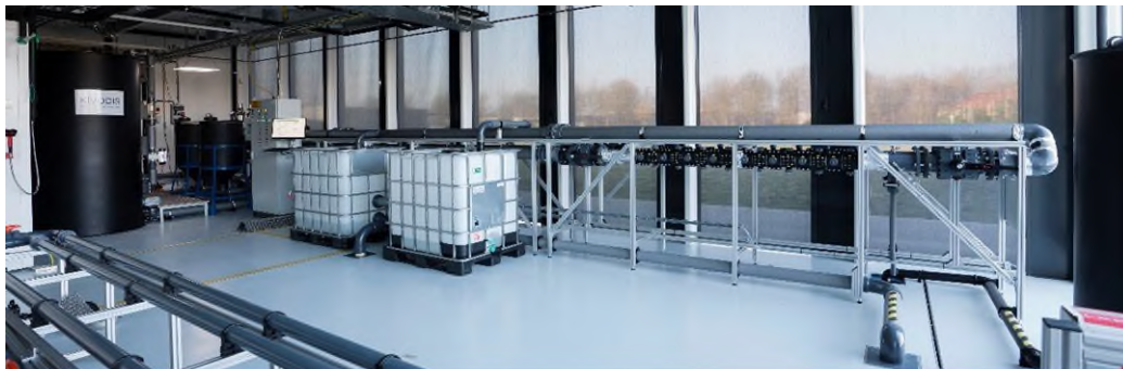
KIVODIS (KWR in vitro distributiesysteem) pilot installation at KWR.
