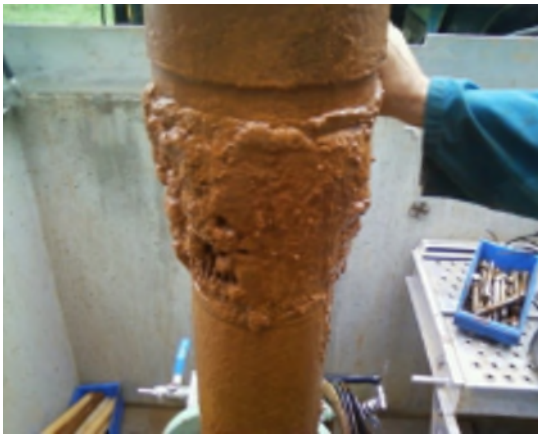
Groundwater wells regularly become clogged by the accumulation of deposits precipitated by the oxidation of iron from the groundwater.
