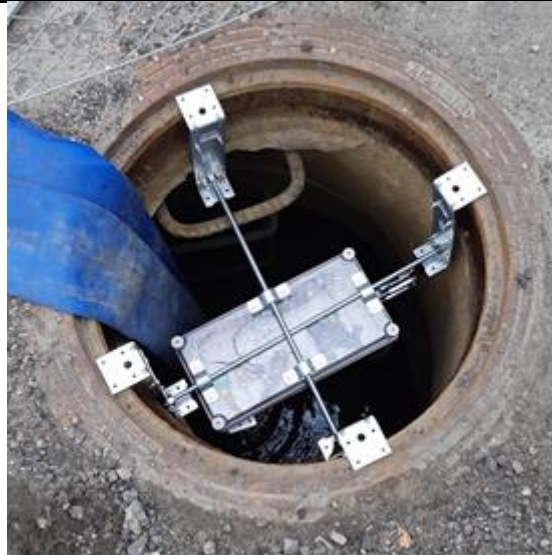
Figure 2: The sensor needs to be robust to withstand the wastewater environment, easy to install and de-install as well as requiring little maintenance.
