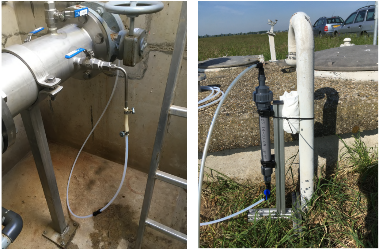
Figure 16: Measuring groundwater abstraction well. Left: connection to the abstraction well. Right: above ground installation
