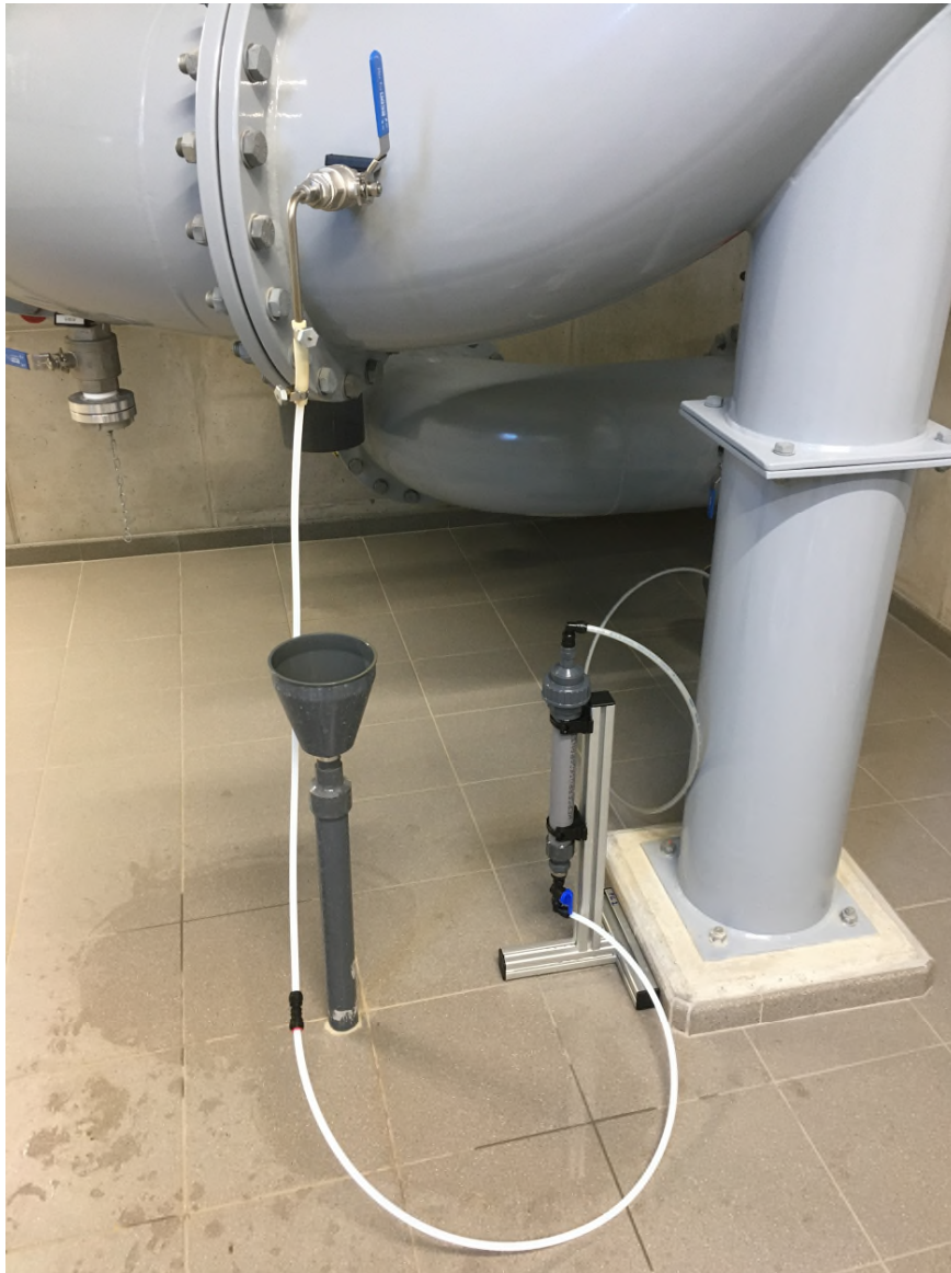
Figure 15: Flow cell installed at one of the pumping stations.
