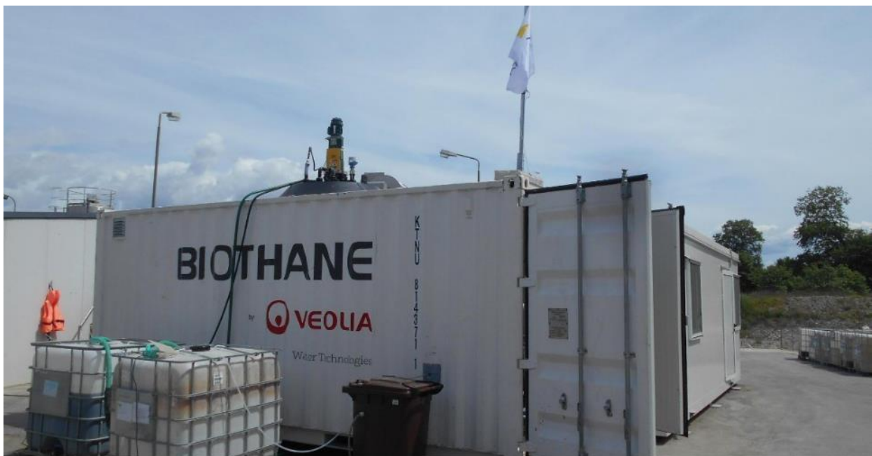
Figure 4 AnSBR containerized Pilot plant
