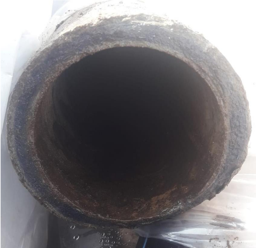
Figure 30 Photograph of AC Test 2 performed in Texel on the Willem van Beierenstraat
