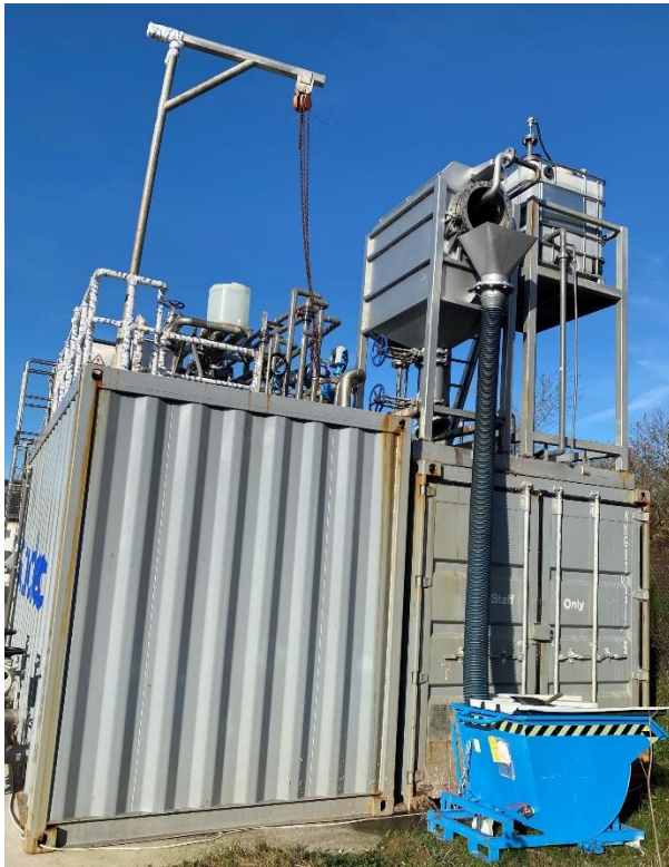
Figure 5 Side view of the pilot plant
