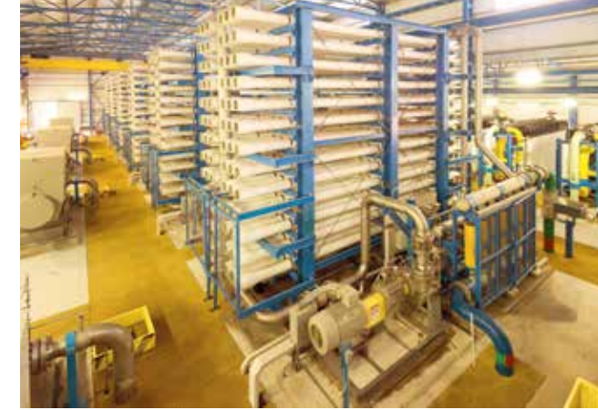
Interior desalination installation
