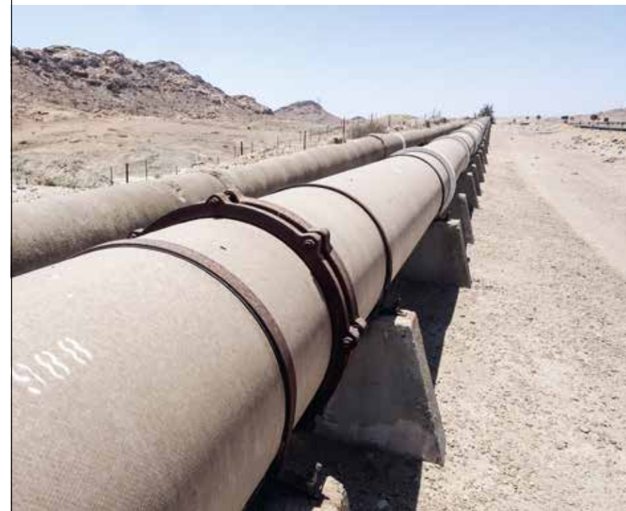
A large gas transport pipeline through the desert
