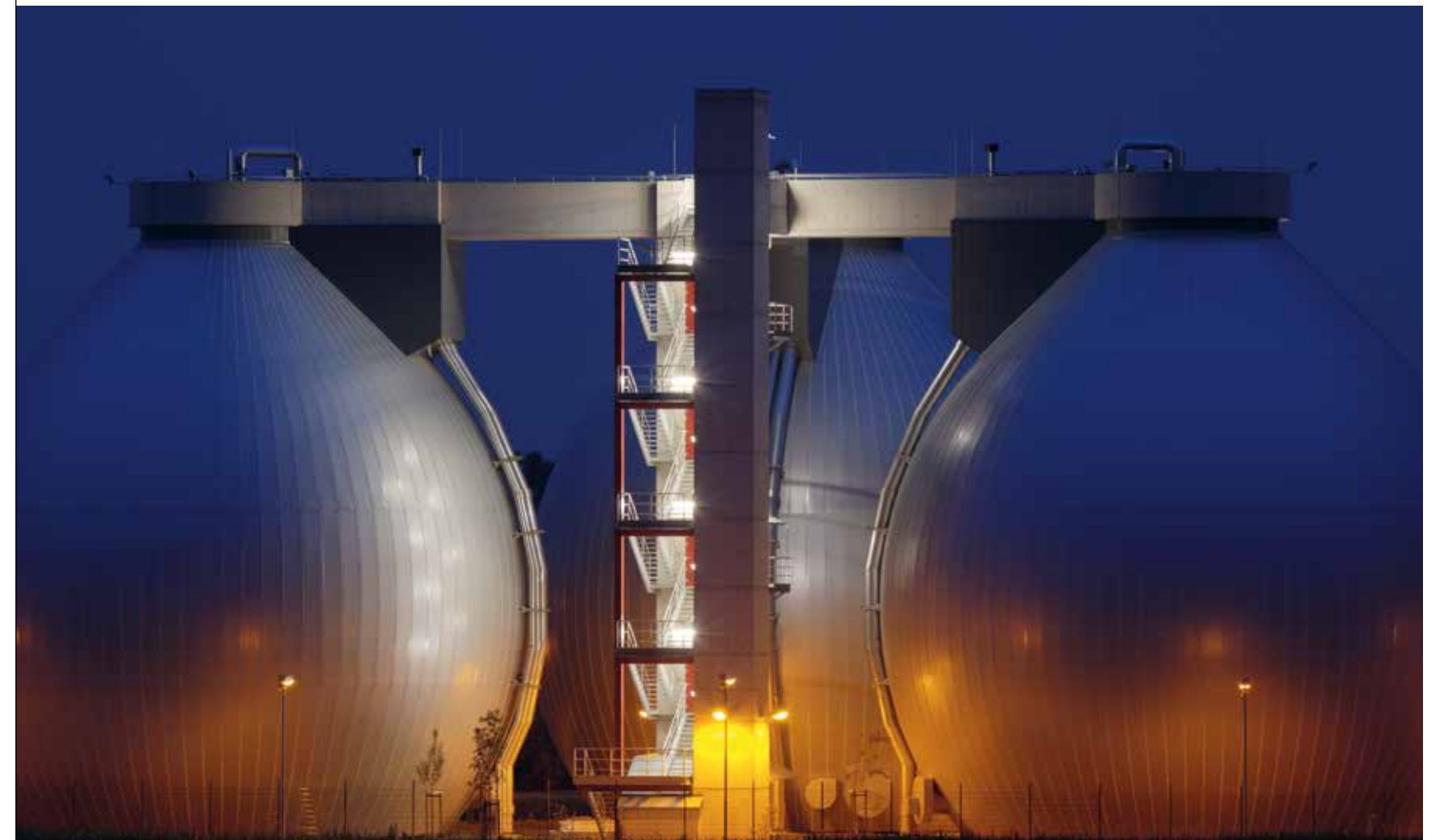
Anaerobic digesters at a wastewater treatment plant
