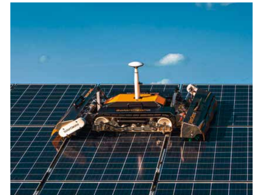
Solar panel robot washer
