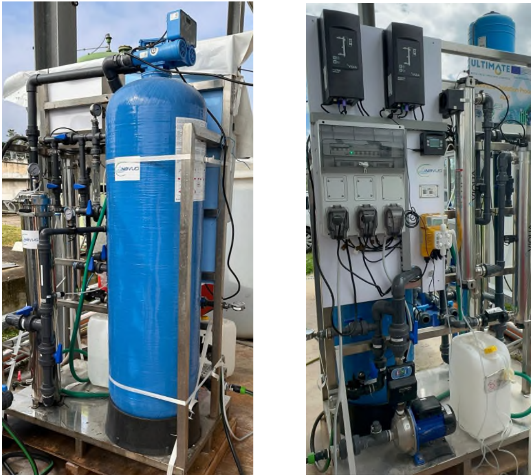
Figure 14. AOP Pilot Plant
