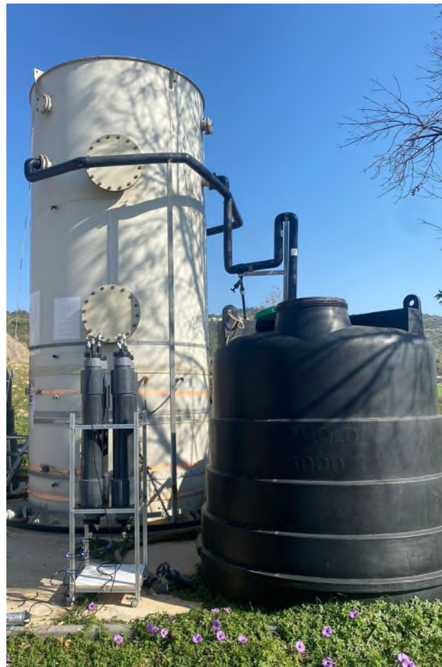
Figure 54 GtG adsorption system in the front side of the AAT at the Karmiel site.
