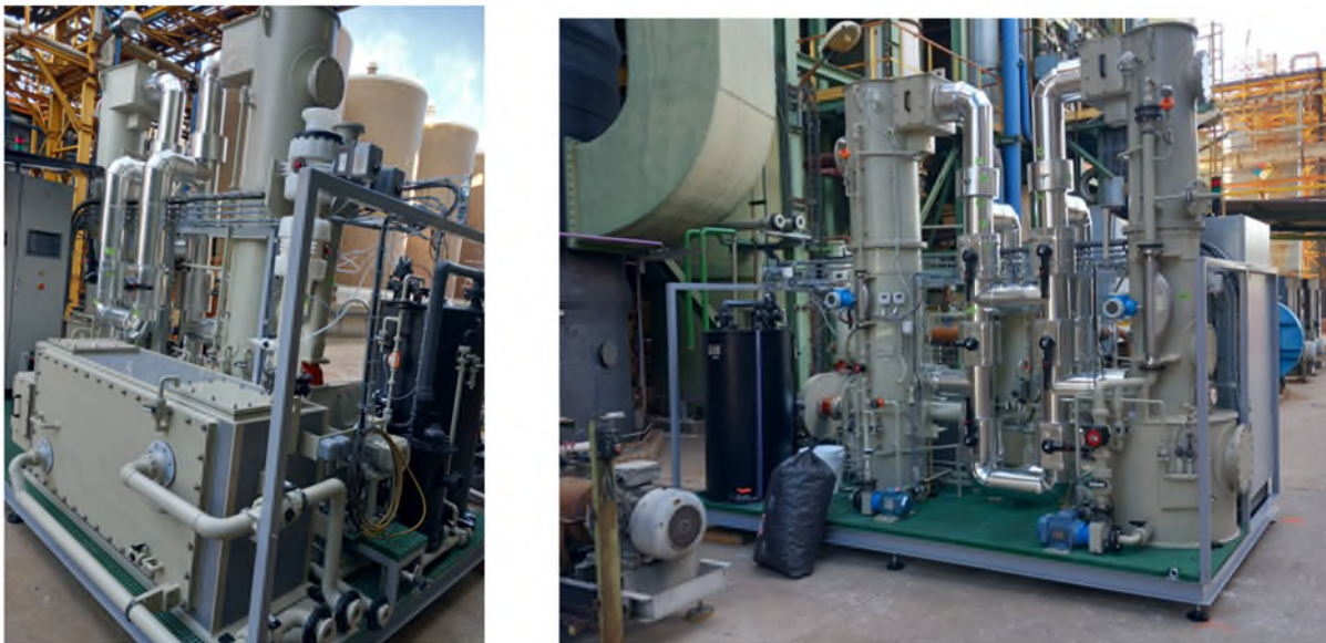
Figure 76: Pictures of the sulfur recovery system.
