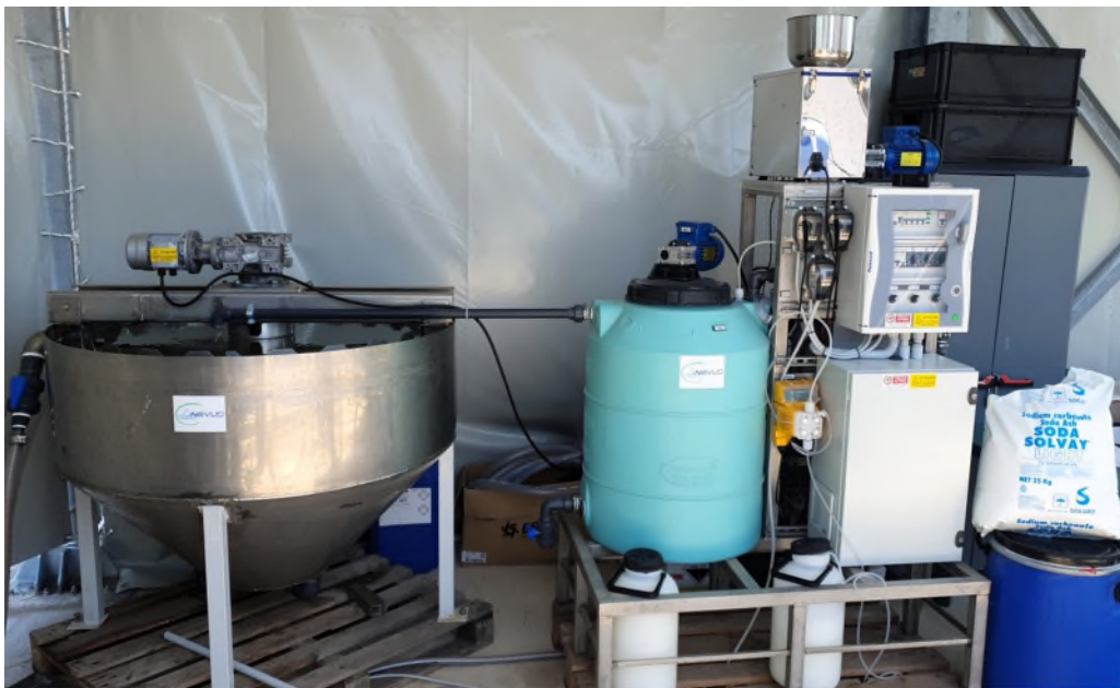
Figure 9 Clariflocculation pilot plant: a) flow diagram; b) picture of the plant.
