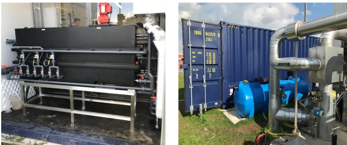
Figure 1 EC (Qstone) Pilot set-up. Left: EC reactor and flocculation units. Right: Containerized pilot and feed tank.
