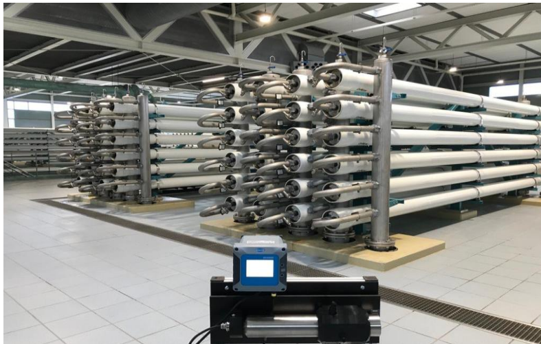
Figure 5 SAC sensor (HACH) installed at Heemskerk, PWN full-scale Ultrafiltration installation.
